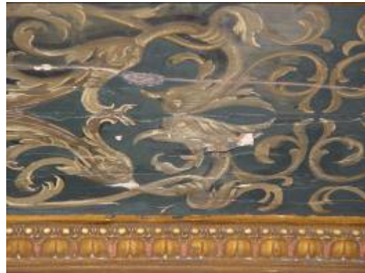
21. Detail of Ceiling Needing Conservation Treatment. A professional conservator will fill and inpaint damaged areas in the design as necessary to unify the visual appearance of this decorative finish.
